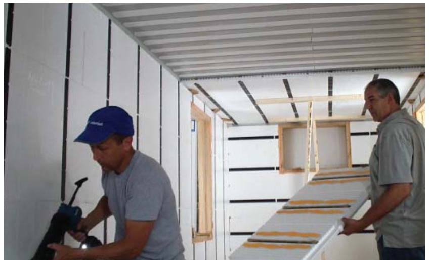
To keep the studs centered in the container, trim off the ends of both panels.
