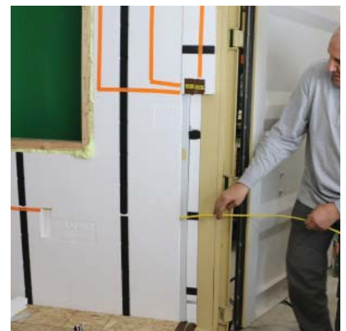
Wire in horizontal raceway.
