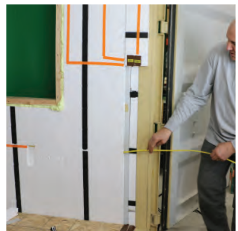
Wire in horizontal raceway.
