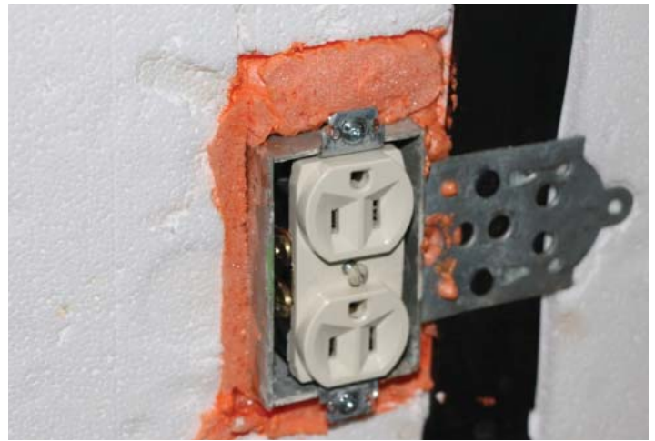
Extended electrical box.
